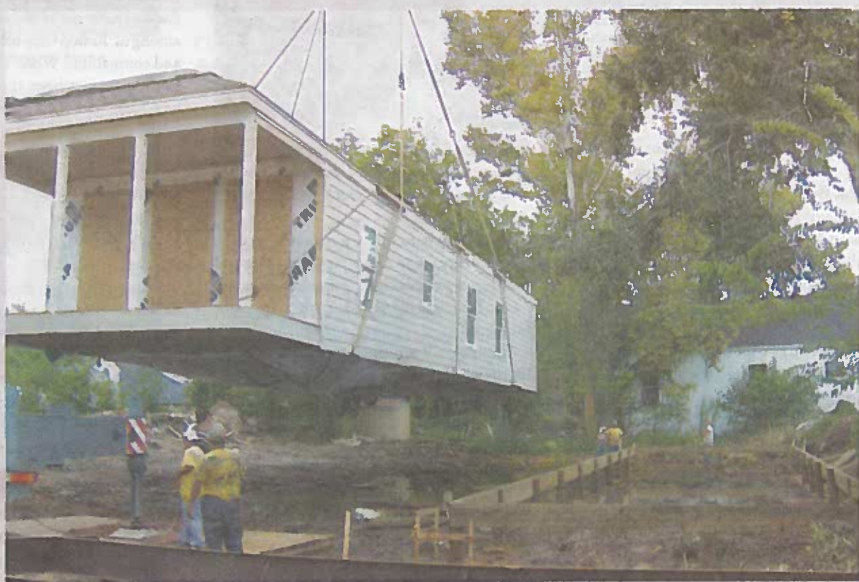
[RIGHT] A crane lifts one of the modular houses from a flatbed truck as workers on the ground direct the structure onto its foundation pilings and secure it in place at 2409 Philip St. [JOHN JOHNSON PHOTOS]
